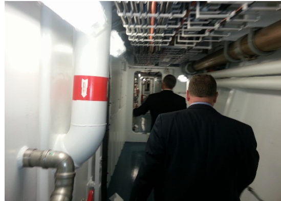
Straight Run Service Piping and Cabling
