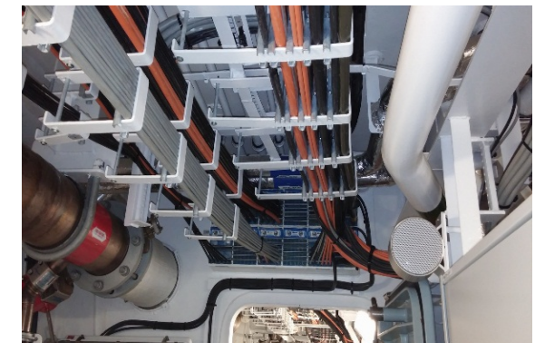
Extra-Large Cabling Tray and Penetrations
